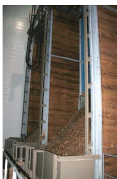
Le stockage de bois © COFELY Services
